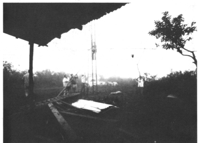
HC5K climbing ladder to hoist the 20 M. beam while crew braces homebrew scuffle
